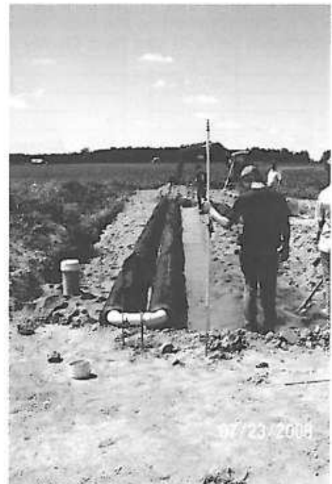
Typical Enviro-Septic® absorption field installation in Van Wert County.
