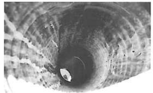
Water accumulated at infiltrative surface
