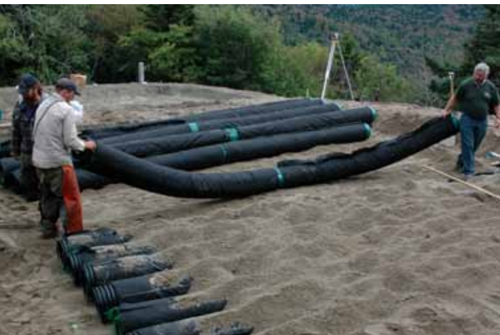
Once the couplers and end caps are in place, the black geotextile is pulled to meet the plastic fitting.
