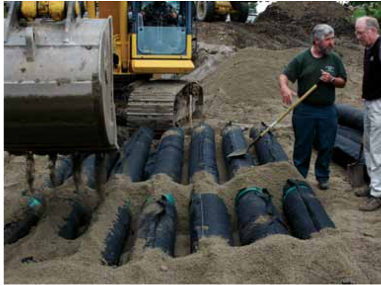
David W. Presby, owner of Presby Environmental, explains how the Enviro-Septic pipe is held in place with the specified system sand during installation of the Mt. Sunapee Lodge wastewater treatment system.
