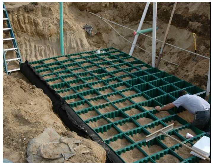
The above photo shows a De-Nyte™ cell array during installation at the Massachusetts Alternative Septic System Test Center in Barnstable, Massachusetts.
