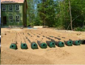
Enviro-Septic® in LEED Home
