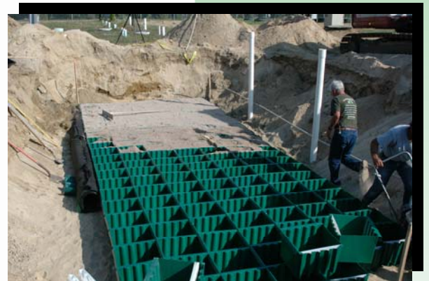
De-Nyte™ Installation at Massachusetts Alternative Septic System Test Center
